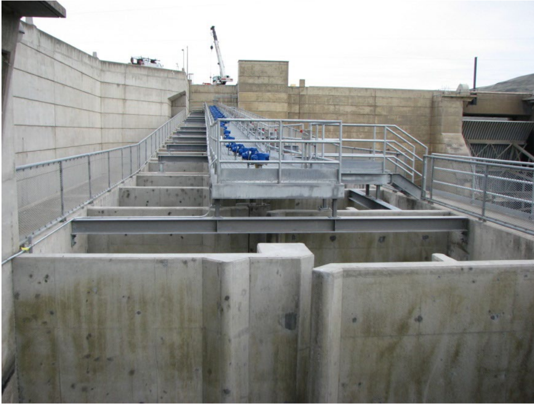
Figure 2-2. John Day North Fish Ladder Slot and Orifice Control Section in 2010, after Rebuild.
